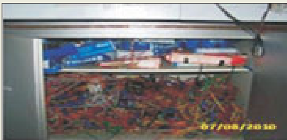
Electrical wires kept without sorting
